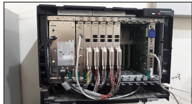
Photographs showing the installed Telephone Exchange System
